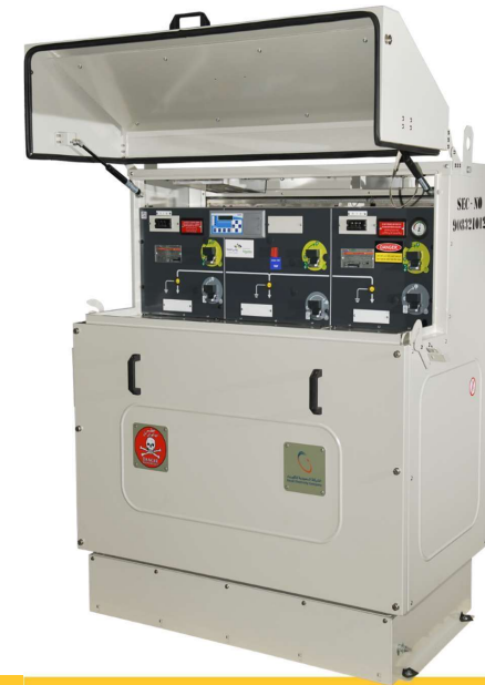
Outdoor 13.8 kV RMU
