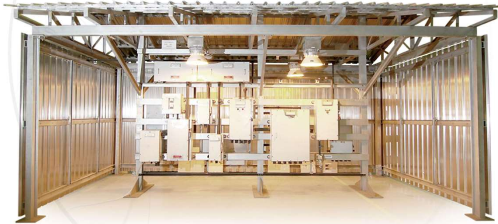
Fenced NEMA-4X Switchrack
