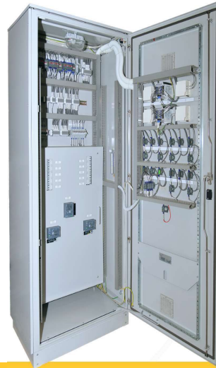
Main Distribution Board
