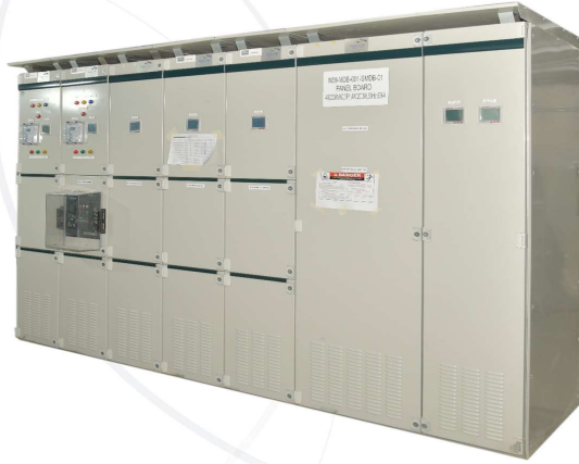
Low Voltage Switchboard
