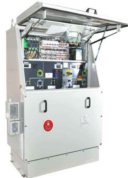
Smart (Automated) 13.8 kV RMU
