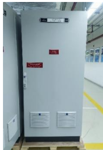
Vibration Monitoring System Cabinet
